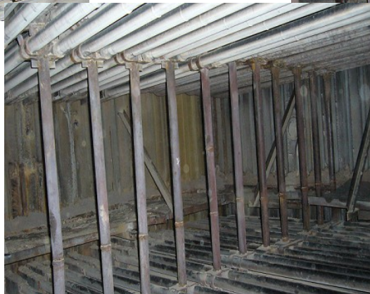
Photographs shows the Expanded Metal Screens (EMS) installed based on the C.A.V.T. measurements
