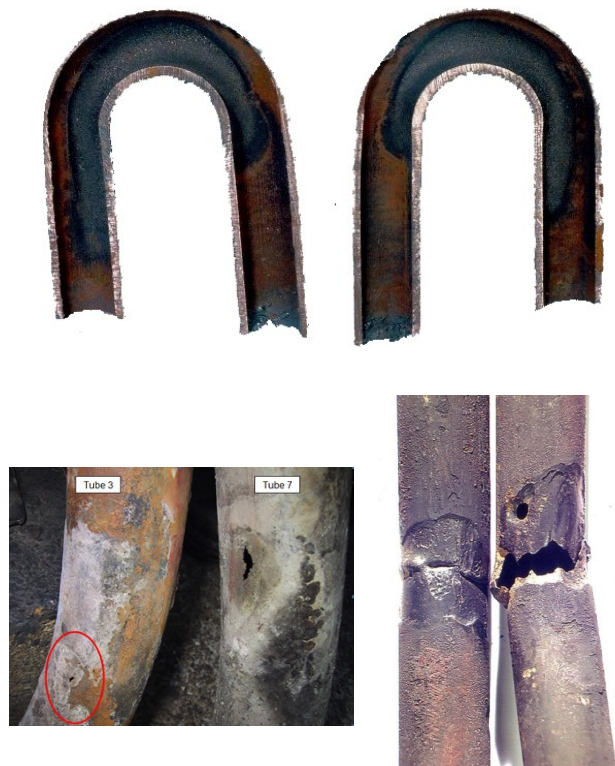
Above Fig. shows the Boiler Tube Leakage pattern
